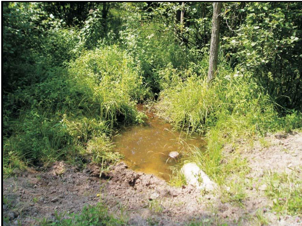
Photograph 39. Outlet culvert on Watercourse 2, downstream of W2. Note the low flow conditions and ill-defined downstream channel reach (July 29, 2004).
